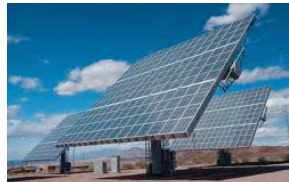
Solar Power Plant Monitoring
